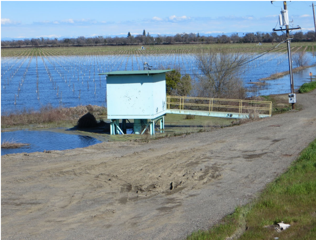
Figure 9. Existing RD 537 pump station
